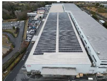
Solar panels at Okayama Plant
