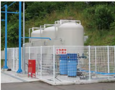
LPG gas tank (Yumoto Factory)
