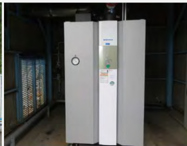
Steam boilers (Yumoto Factory)
